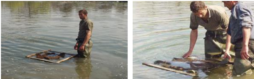
Figure 2 (a-b). Installation of mattresses for directed reproduction of the saddle (original photo)
