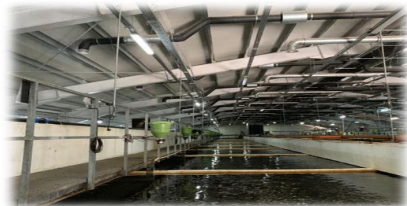
Figure 3.1 - Recirculating Aquaculture System (RAS) in Indoor Facilities
