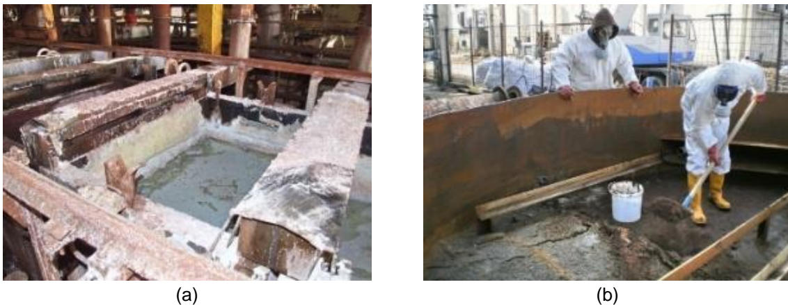
Figure 3.1. Images during decommissioning of the electrolysis plant and decontamination of the work area: (a) decommissioned electrolysis plant and (b) decontamination of the work area (source: adapted according to [Sloată and Ene, 2017a, b])
