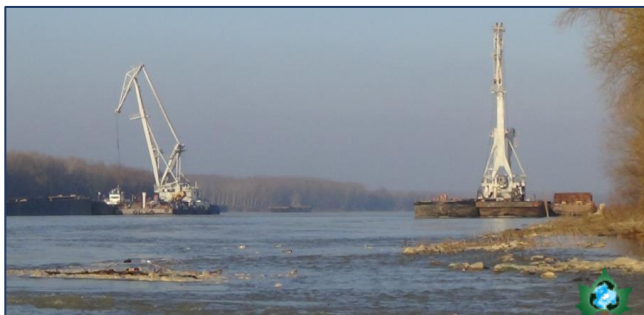
Figure 35. Construction of hydrotechnical structures to improve navigation conditions on the Danube (INCDPM, 2015)
